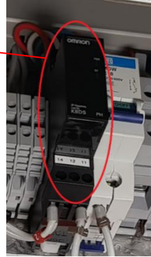
PHASE DETECT RELAY
